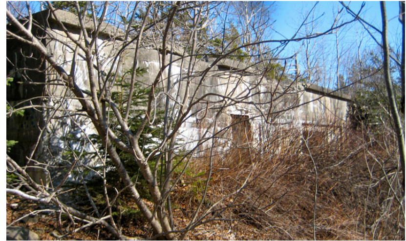
Concrete structures in variable states of decay.
