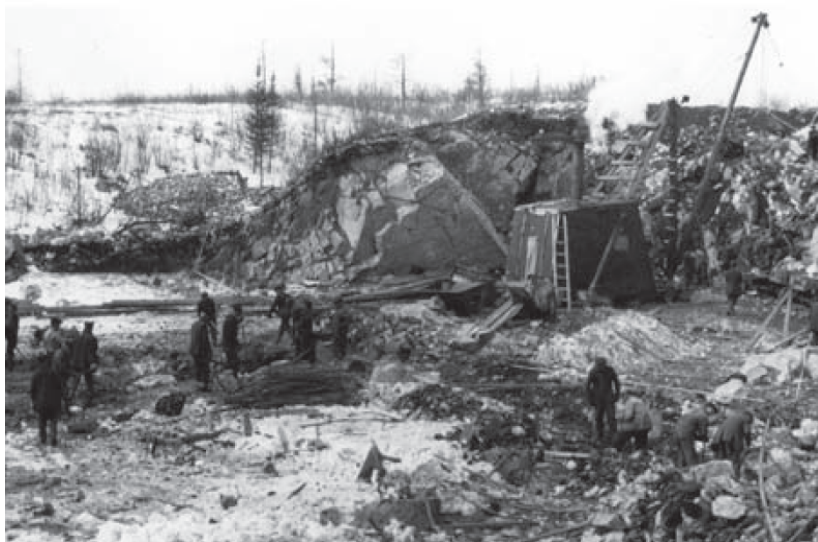
Excavating granite bedrock for the construction of the military barracks (PHOTO: CFJIC RE 84-171, from Sarty and Ellis, 2009)
